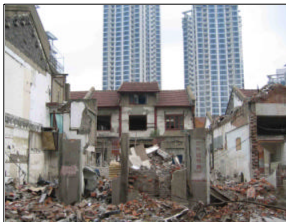
Old buildings come down as new ones go up to make space for Shanghai's 20 million residents.
